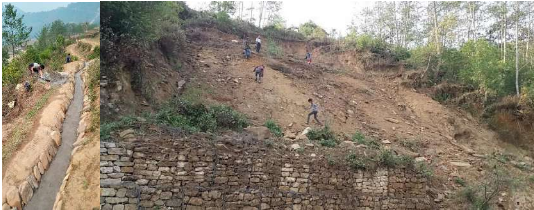
(Crack filling with Green turfing topping, Drainage canal in the left and the landslide in the right)
